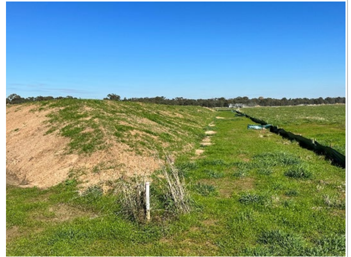
Photo 14: Shaped and formed stockpile with sediment fence and located away from driplines of trees
